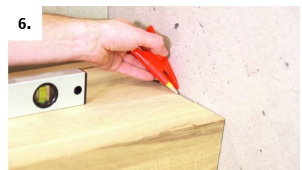
6. Mark the staircase steps on the construction site and, where necessary, adapt them to the spatial situation in a user-friendly way.
